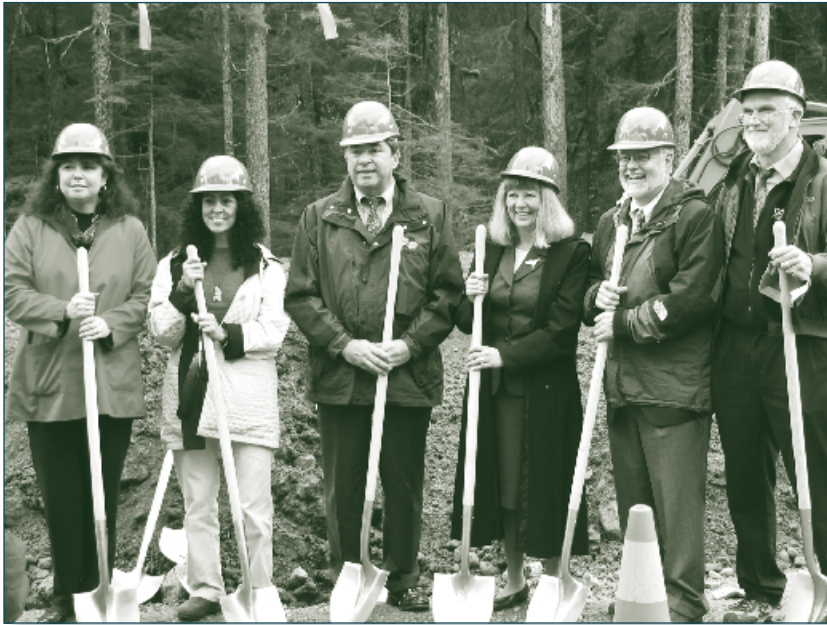
Breaking ground for the Juneau Youth Services residential treatment facility are, from left to right, Connie McKenzie, congressional delegation staff representative; Amalia Monreal, Vice President of the Juneau Youth Services Board of Directors; Ken Brewer, President and CEO for SEARHC; Karleen Jackson, DHSS Commissioner; John Pugh, Chair, Alaska Mental Health Trust Authority; Walter Majoros, Executive Director, Juneau Youth Services.
